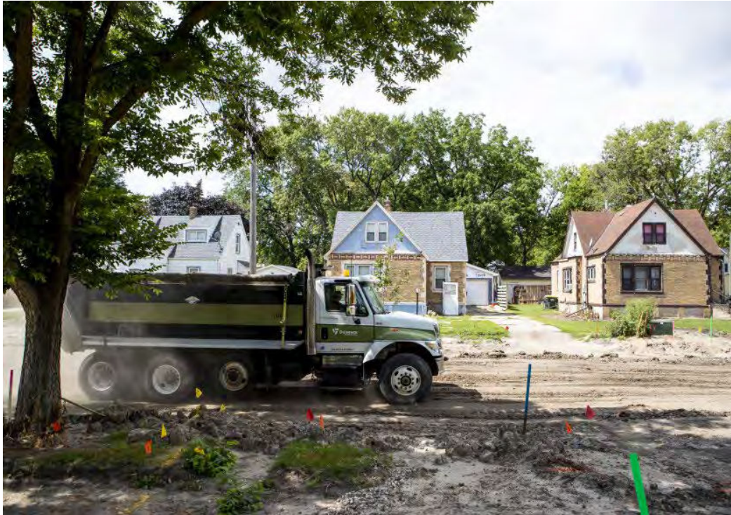
A driver for Duinick Inc. hauls away dirt along Charlotte Street Southeast road construction in Willmar on Tuesday, Aug. 16, 2022.
