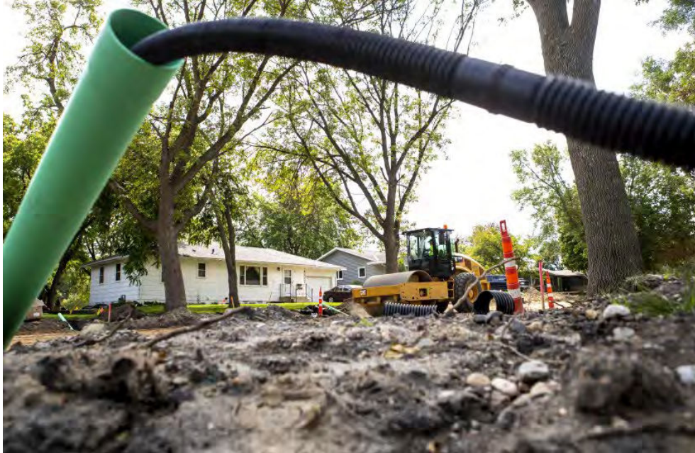
A worker uses a road roller to compact new road material deposited along Sixth Street Southwest on Tuesday, Aug. 16, 2022.
